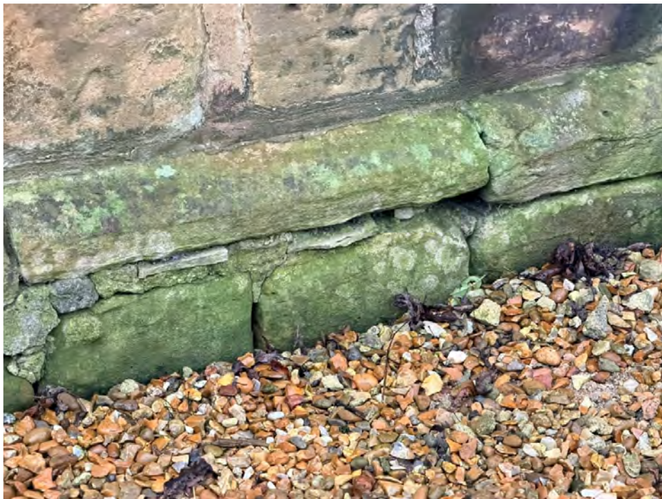
OPEN JOINTS AND ALGAE STAINING ON NORTH PLINTH
