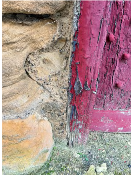
MORTAR REPAIRS AROUND DOOR ALSO ERODING
