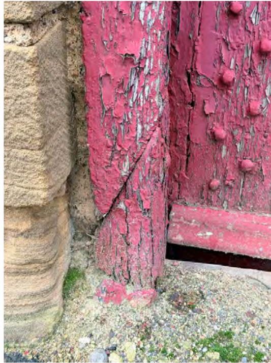
DETERIORATED FRAME TO WEST ELEVATION DOOR
