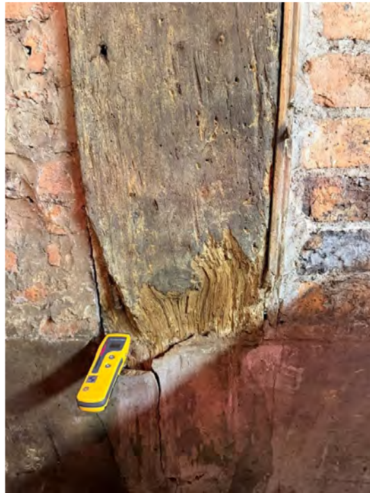
HIG MOISTURE READINGS IN TIMBER TO GROUND FLOOR PARTITION
