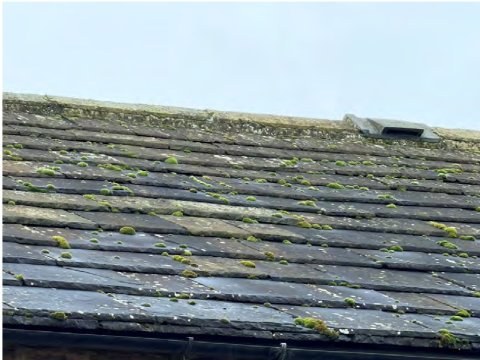
MOSS TO EAST ROOF SLOPE
