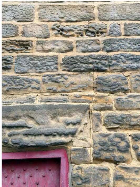
HAIRLINE CRACKING ON SOUTH ELEVATION ADJACENT TO BULGE
