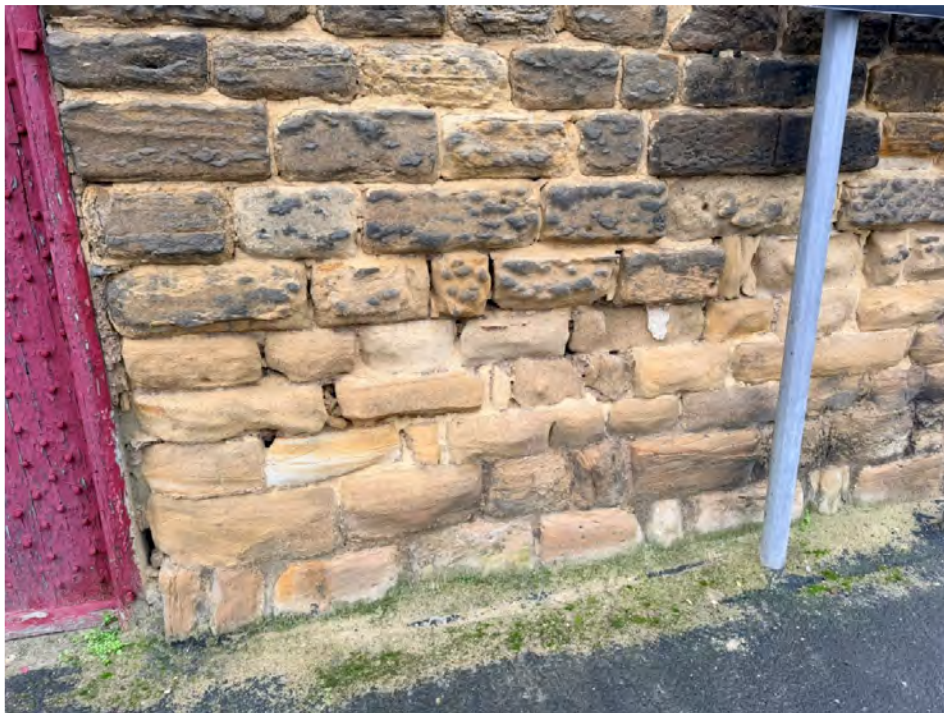
ERODED STONE AND OPEN JOINTS ON WEST ELEVATION
