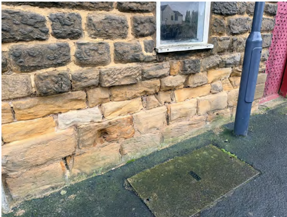
EROSION TO BASE OF WALL ON WEST ELEVATION
