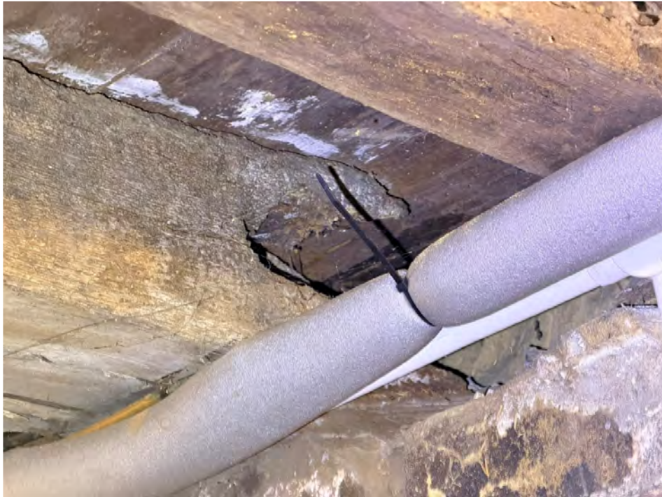
DECAYED FLOOR JOIST ENDS DUE TO DAMPNESS AND INSECT ATTACK
