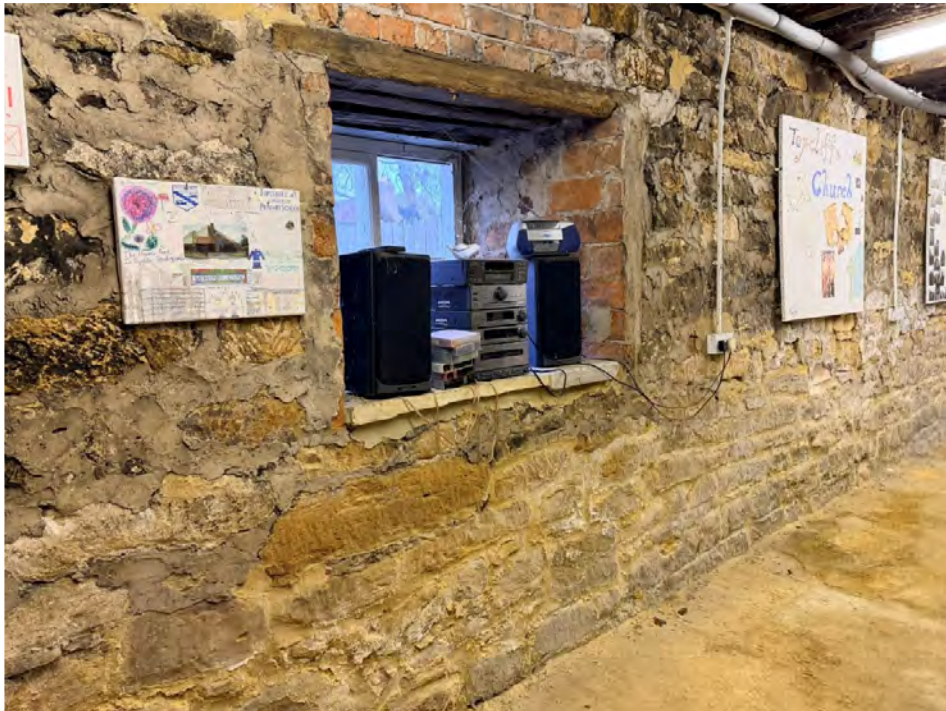
SALT STAINING AND DAMPNESS TO EXTERNAL WALL
