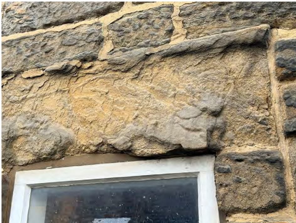
WEATHERED WINDOW HEAD ON WEST ELEVATION
