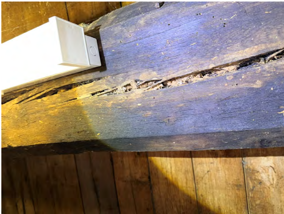
SIGNIFICANT SHAKE IN FLOOR TIMBER
