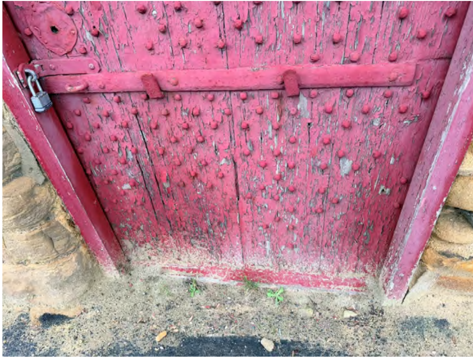
AGED AND DETERIORATED DOOR TO SOUTH ELEVATION
