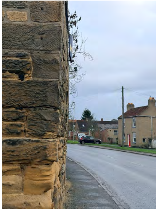
DEFLECTION AND BULGING ON SOUTH WALL
