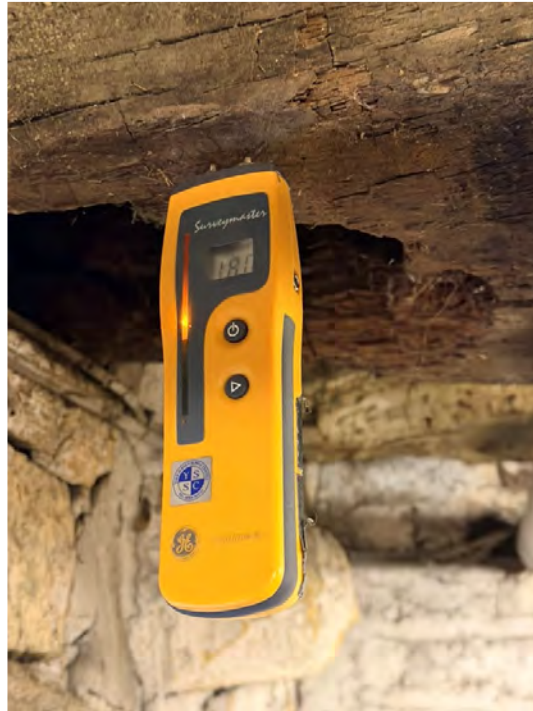
MODERATE MOISTURE READINGS IN FIRST FLOOR TIMBERS
