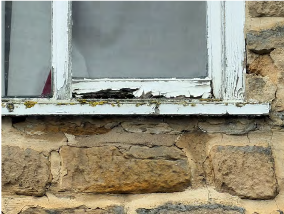
DECAYED TIMBER TO WINDOWS
