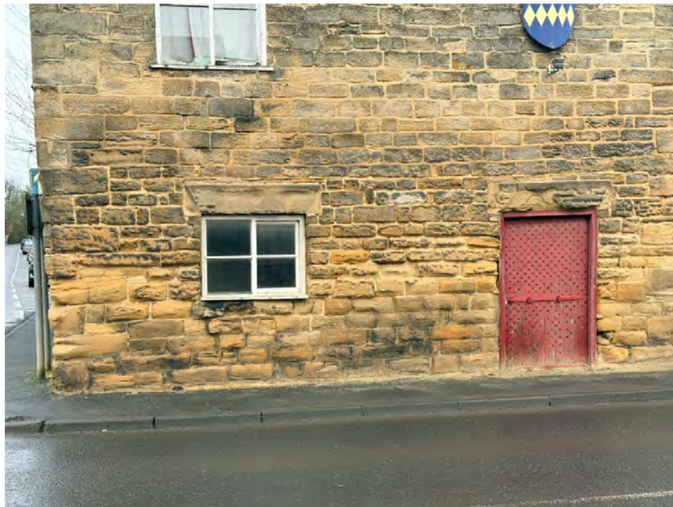
EROSION AND BLACKENING ON SOUTH ELEVATION
