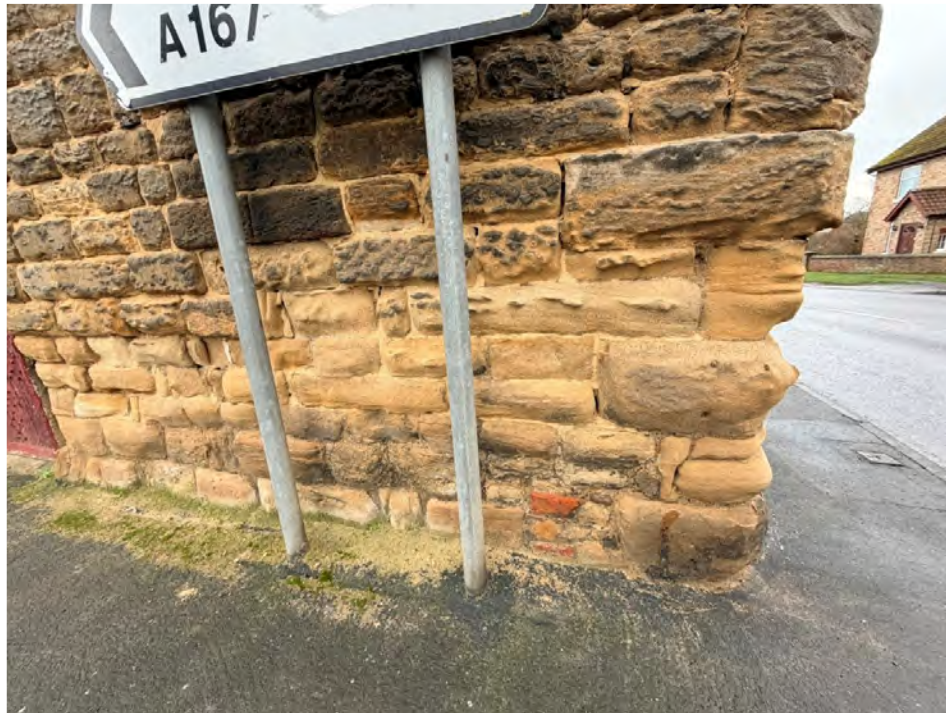
SIGNIFICANT EROSION AT LOW LWVEL TO SOUTH WEST CORNER
