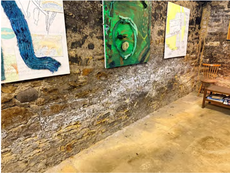
SALT STAINING AND DAMPNESS TO DIVIDING WALL
