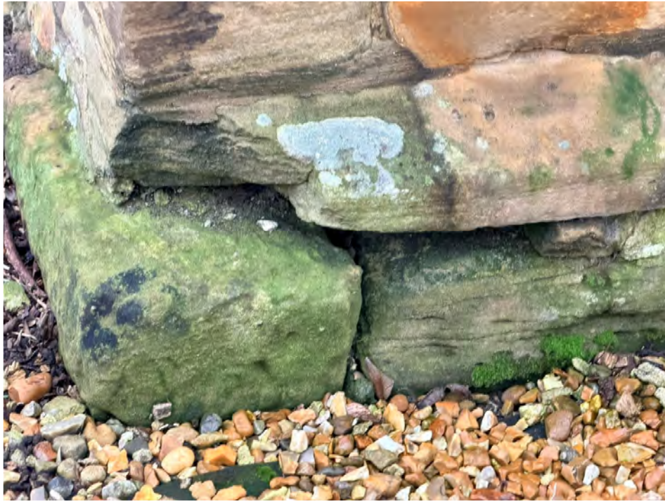
OPEN JOINTS TO NORTH ELEVATION PLINTH
