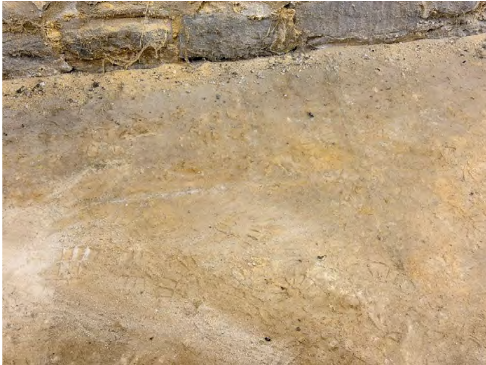
STAINING AND DUSTING OF DAMP FLOOR SLABS
