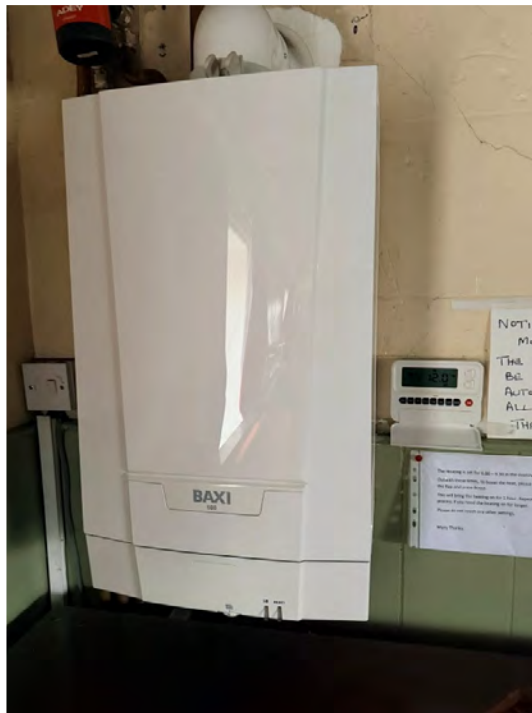
BAXI BOILER LOCATED ON FIRST FLOOR
