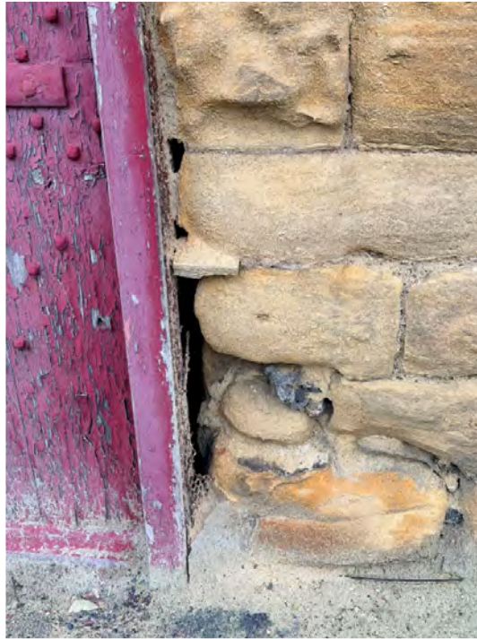
SIGNIFICANT EROSION AROUND SOUTH DOOR LEAVING LARGE GAP
