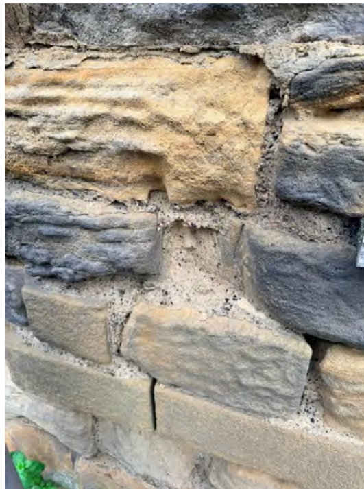
ERODED STONE AND POINTING
