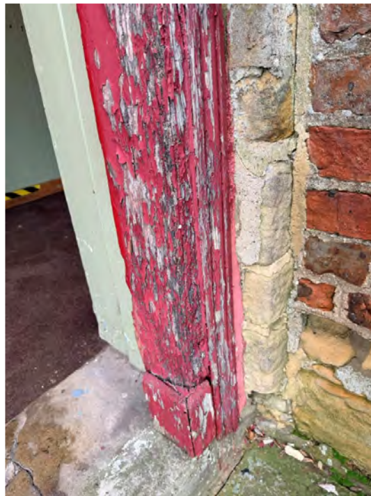
DETERIORATED FRAME TO SNOOKER CLUB DOOR
