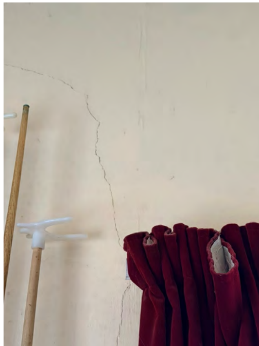
HAIRLINE CRACKING ON WEST WALL
