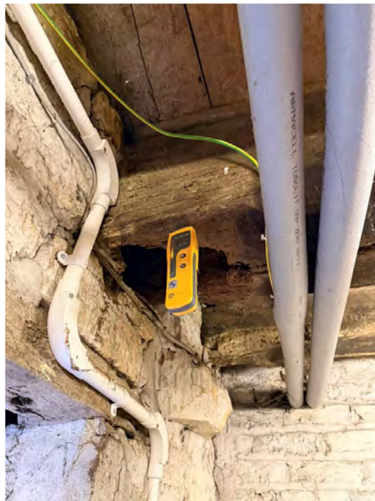
MODERATE MOISTURE READINGS IN FIRST FLOOR TIMBERS
