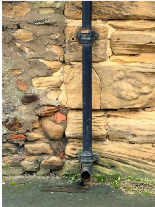
RAINWATER PIPE ON WEST ELEVATION WITH CORROSION AT JOINTS
