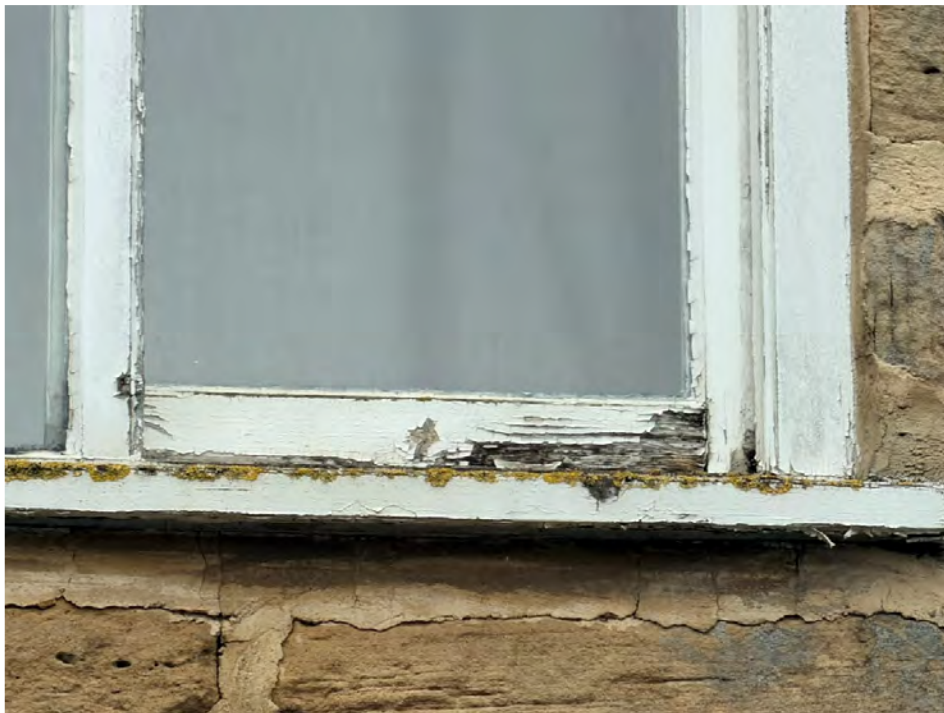
DECAYED TIMBER TO WINDOWS
