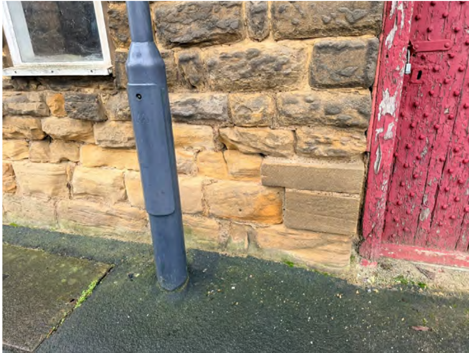
ERODED STONEMWORK AND REPLACEMENTS ON WEST ELEVATION
