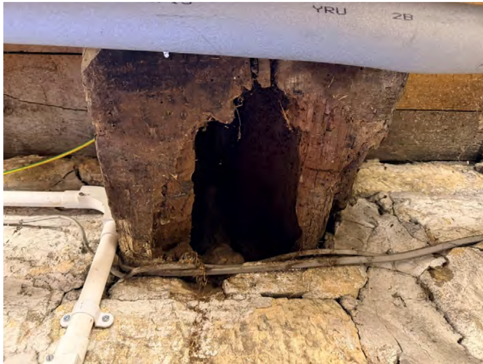
DECAYED FLOOR JOISTS ENDS DUE TO DAMPNESS AND INSECT ATTACK
