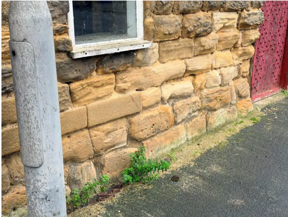
ERODED STONEMWORK AND RECENT REPLACEMENTS ON WEST ELEVATION
