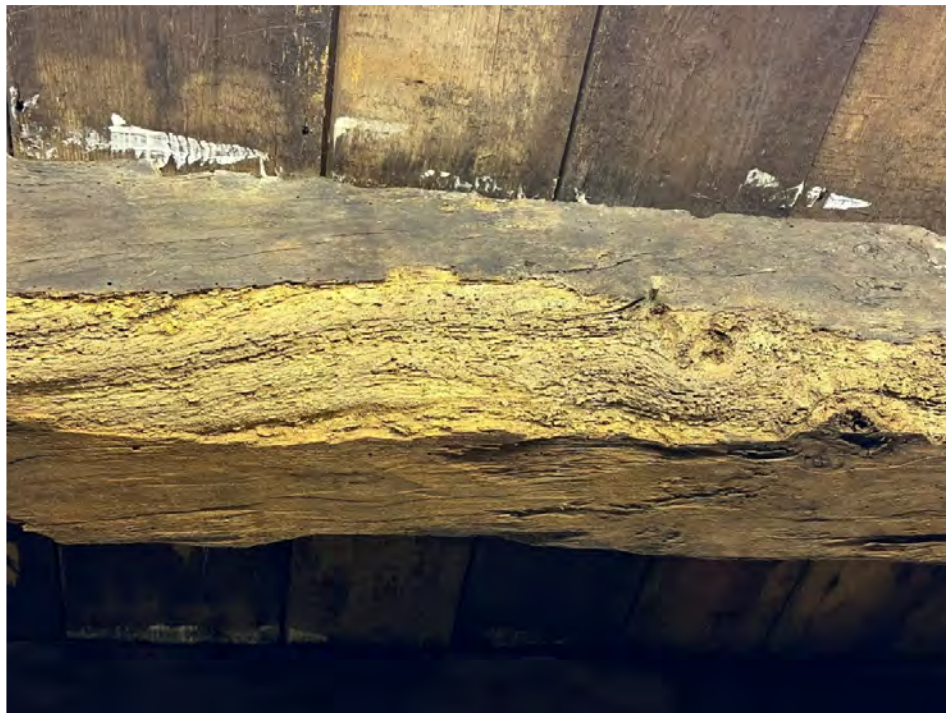
DAMAGED RESULTING FROM WOOD BORING INSECT ATTACK
