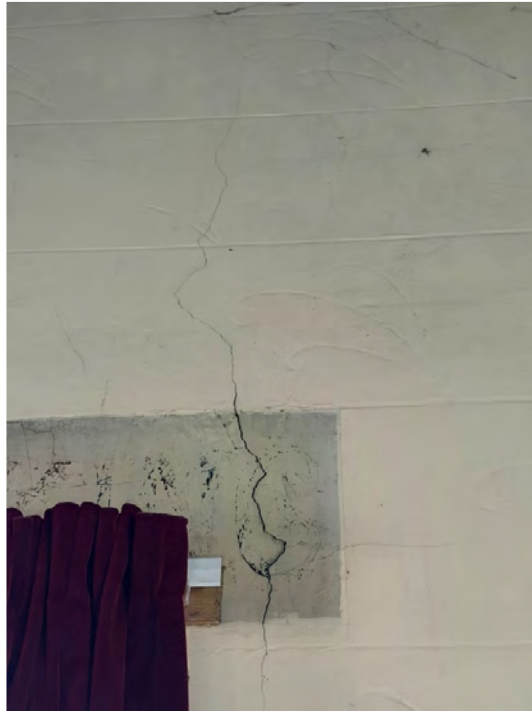
HAIRLINE CRACKING IN PLASTER TO NORTH WALL
