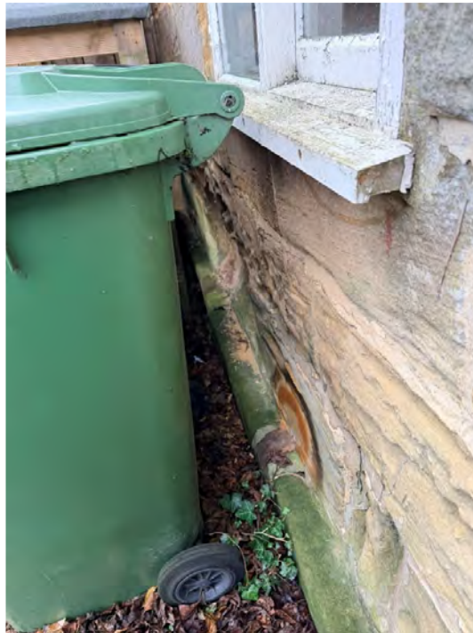
EROSION AT LOW LEVEL ON EAST ELEVATION
